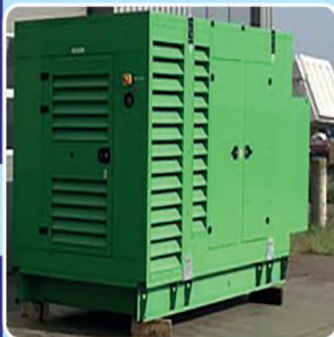
Generator; Brand: Doosan; Capacity: 490 KVA
