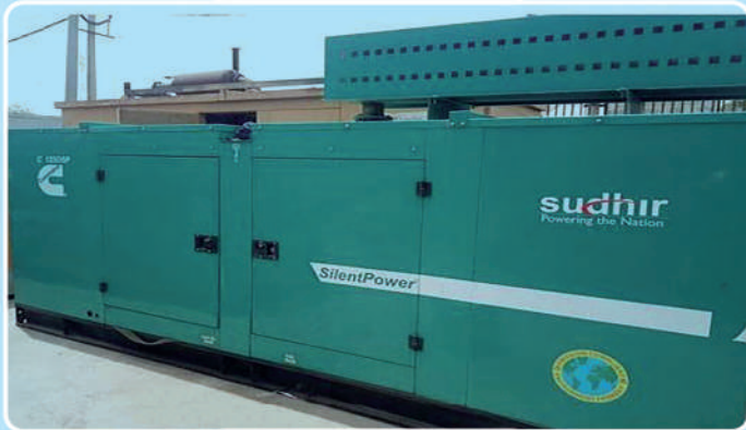
Generator; Brand: Cummins; Capacity: 1000 KVA
