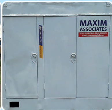
Generator; Brand: Perkins; Capacity: 350 KVA
