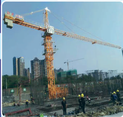
Tower Crane; Brand: Dahan; Model: QTZ100, Boom-60m, Capacity: Bottom-6 Ton, Tip(55m)-1.7 Ton, Manufacture Year: 2014
