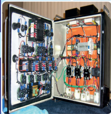
Panel Internal Wiring
