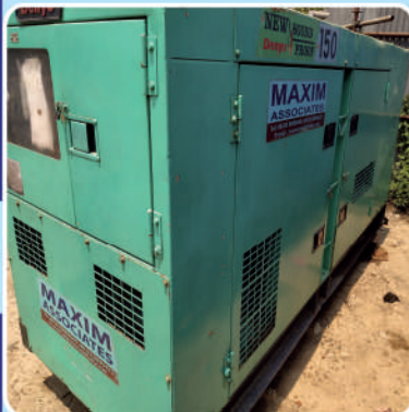
Generator; Brand: Denyo; Capacity: 150 KVA
