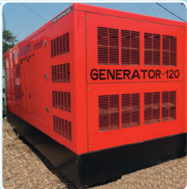
Generator; Brand: Himonsa; Capacity: 550 KVA
