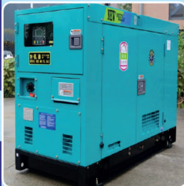
Generator; Brand: Denyo; Capacity: 100 KVA
