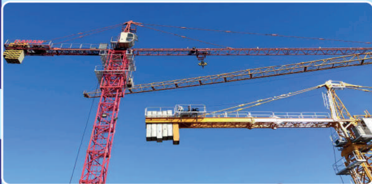
Tower Crane; Brand: Dahan; Model: QTZ63, Boom-50m; Capacity: Bottom-5 Ton, Tip (50m)-1.3 Ton; Manufacture Year: 2014
