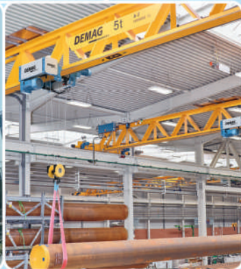
Overhead Crane; Brand: Demag; Model: A-2 14990292; Capacity: 5 Ton; Manufacture Year: 2014
