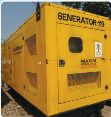
Generator; Brand: Komatsu; Capacity: 550 KVA
